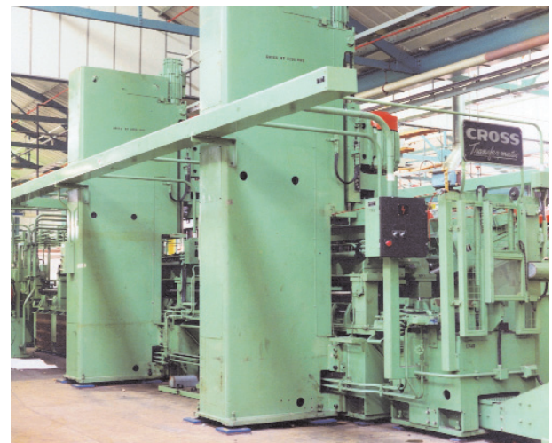
Diesel engine cylinder block transfer line installed on Jackmounts.
