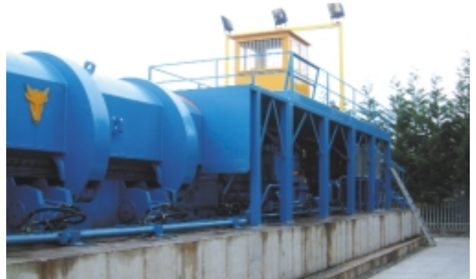
Metal recycling and crushing machine on ISOMAT/FVF isolated foundation
