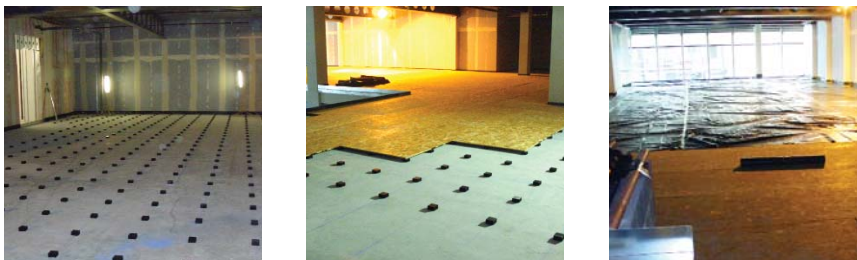
Installation sequence for a gym being constructed within a city centre office building.
